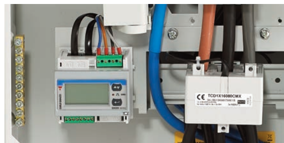
One dual channel standard meter (via two separate block CTs) for separate lighting and power readings
